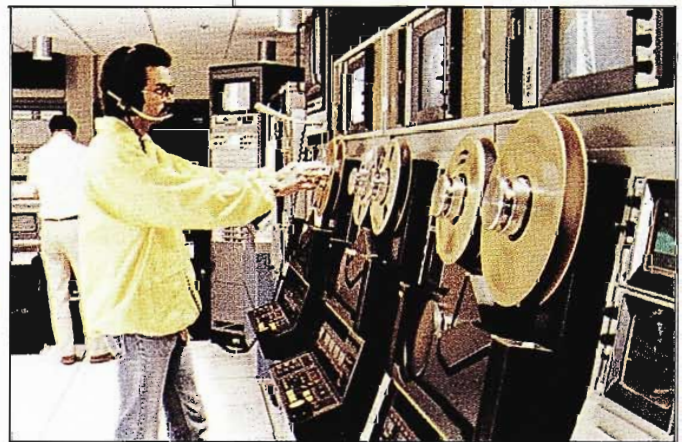
Multi-format tape facility includes TR-800 one-inch VTRs, quad machines and videocassette units.
